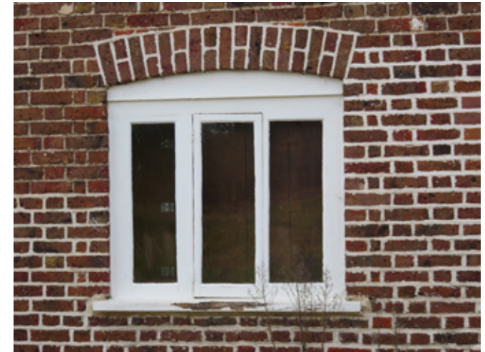
Figure 87 Rotting window sill
