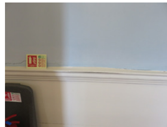
Figure 83 Example of the cracking in the central room
