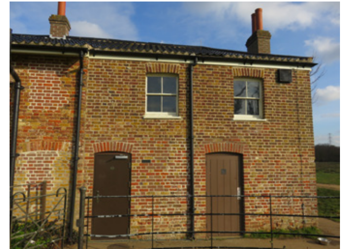
Figure 90 The estate railings have failed paintwork partly because they are climbed on, especially near the WCs
