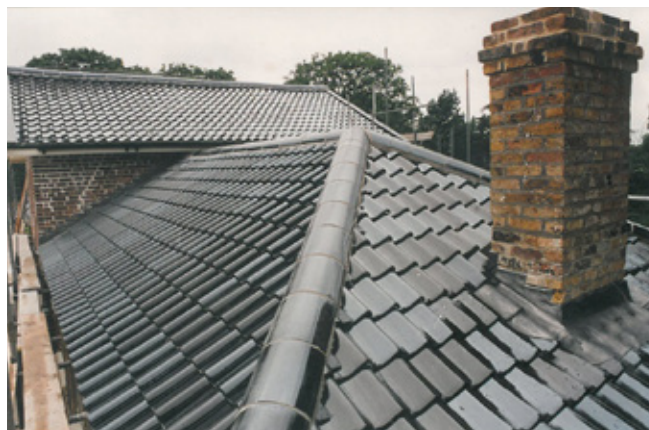
Figure 68 New roof tiles in the 1990s. Reproduced with permission of the City of London Corporation.
