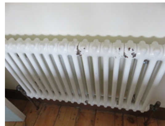
Figure 84 There are internal decorative failures such as to several of the radiators
