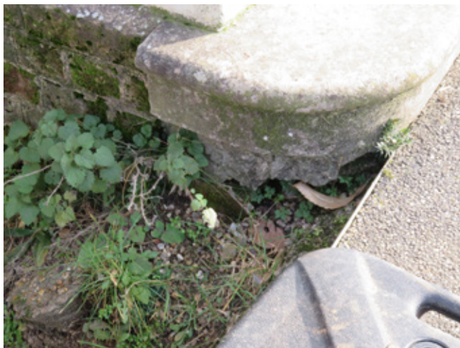
Figure 88 Erosion under the main steps
