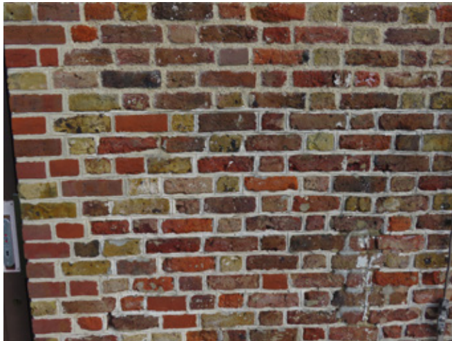
Figure 85 Some of the pointing is drude and there are small areas of cementitious mortar
