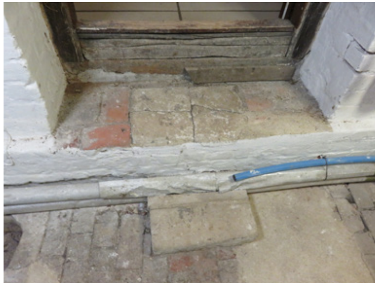
Figure 23 Threshold between the central room on the lower-ground floor and the brick vault.
