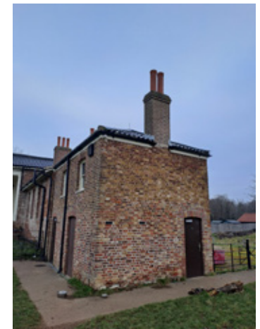
Figure 09 The south elevation of The Temple, showing the modern door providing entry to the men's public toilets at lower-ground floor level
