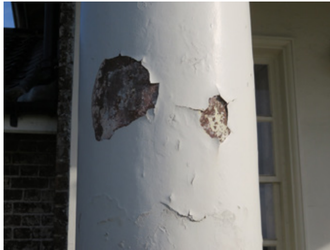
Figure 89 Failing paintwork to the columns
