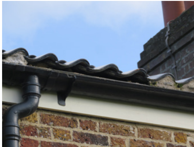
Figure 86 Failed mortar ends to the roof tiles
